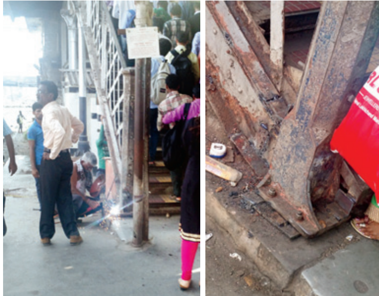
The hurriedly carried out work at Parel station on Thursday. The passenger flow at Parel has increased significantly, but the facilities there have not been upgraded
